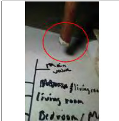
A small amount of water was dripping from this tube.
